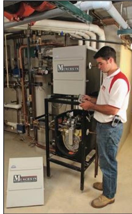
The integrated boiler management system that controls the two stacked Munchkin boilers switches from unit to unit to assure equal run times, so that neither becomes the workhorse of the system.
