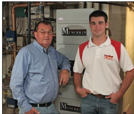
Installer Craig Ouimette (right) and Fred Miller of Miller Construction with the two Munchkin boilers that support the radiant heating system at Pine Ridge Wisconsin Rapids
