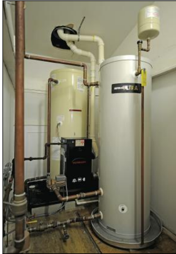
A Voyager Stainless Steel Water Heater, with an input of 199,000 BTU and 45 gallons of internal storage (background), is coupled with an 80-gallon SuperStor Ultra storage tank (foreground) to provide hot water to 16 guest rooms.
