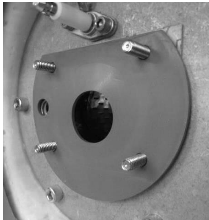
Figure 7 – LP Burner Flange
