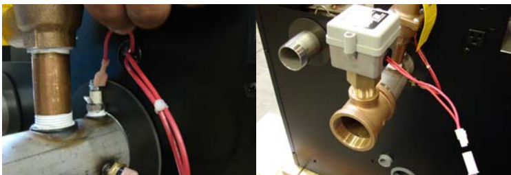
4. Disconnect red wire on the Low Water Cut off Probe and connect it to the red wire from the wire harness (included in kit)
